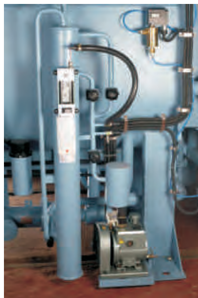
The Purge System
