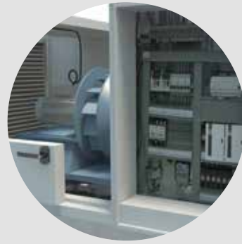
Segregated cable channel and factory-installed control panel
